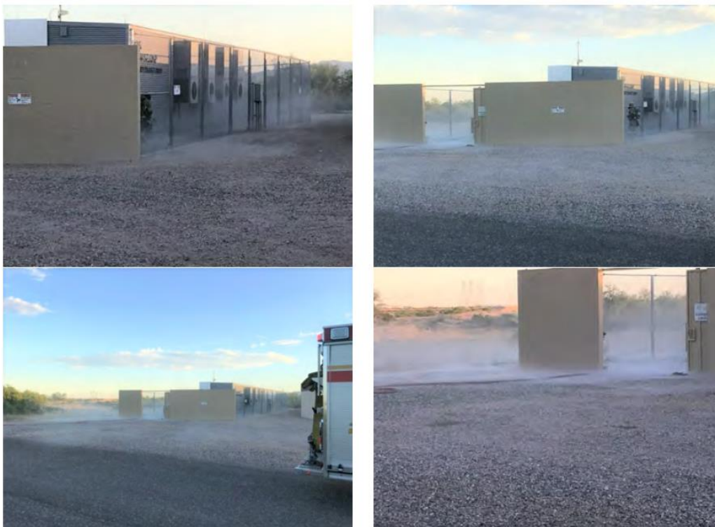
Figure 5.1 Photos of ESS Prior to Explosion (McKinnon, DeCrane and Kerber, 2020)
