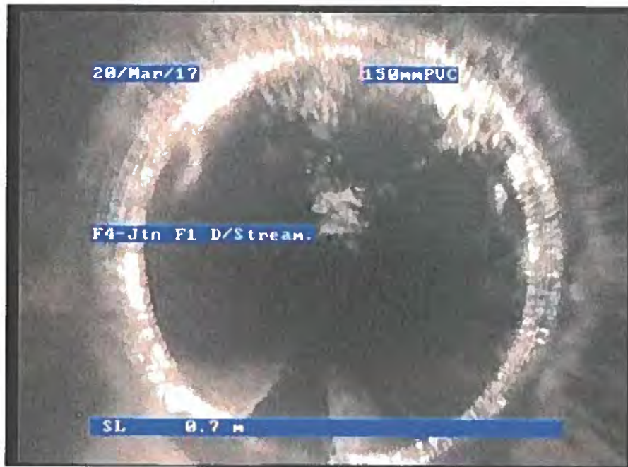
F4X_e26cb627-f968-4340-82cf-58f2f71bbdff_20170321_122719_308.jpg, 00:00:10, 1.00m Joint displaced, large
