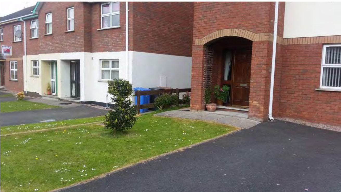
Plate 6 Relative Movement between House 11 and external areas
