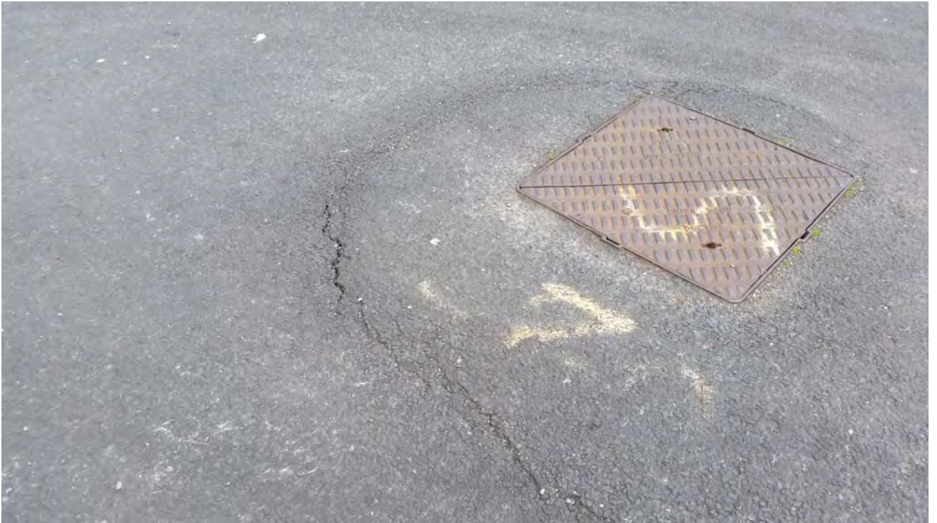
Plate 15 Reflective cracking in road at MH S4
