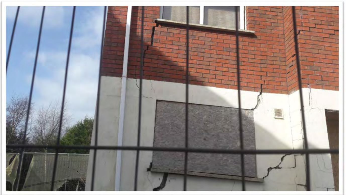
Plate 10 Severe Cracking at House Nr 21
