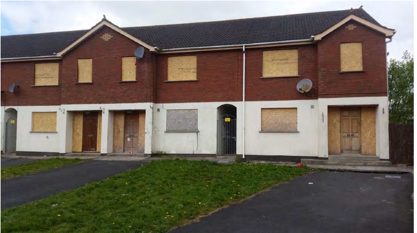
Plate 7 Severe Cracking House Nr's 17 to 21
