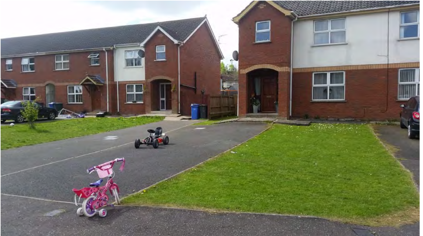
Plate 13 Differential Settlement Between House Nr 23 and external areas
