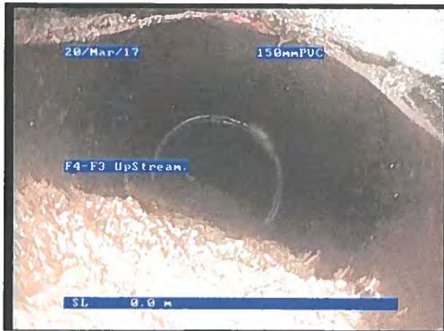
F3X_bbf30af-c854-41fa-af5d-d1cd1aac91b_20170321_122406_687.jpg, 00:00:01, 0.00m Settled deposits, hard or compacted, 40% cross-sectional area loss
