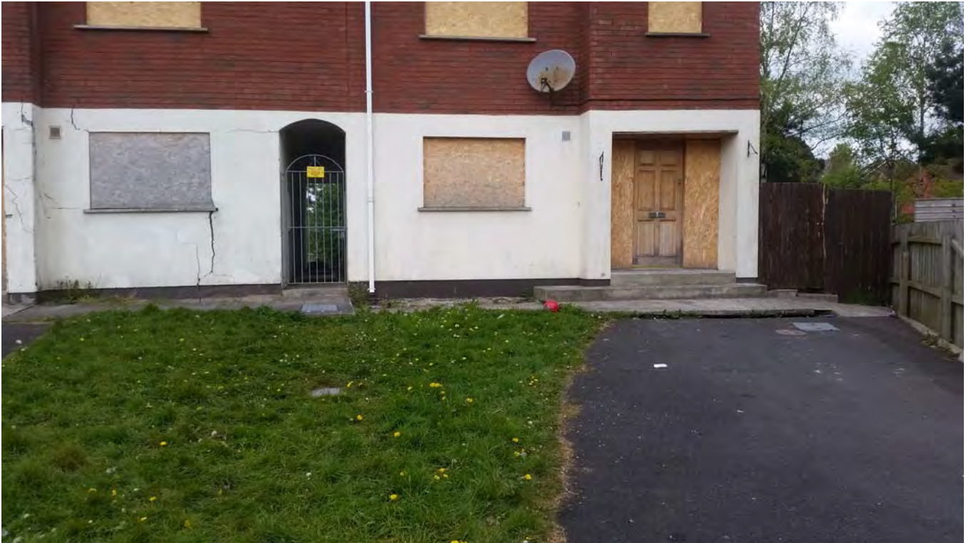
Plate 9 Differential Settlement at House Nr 17
